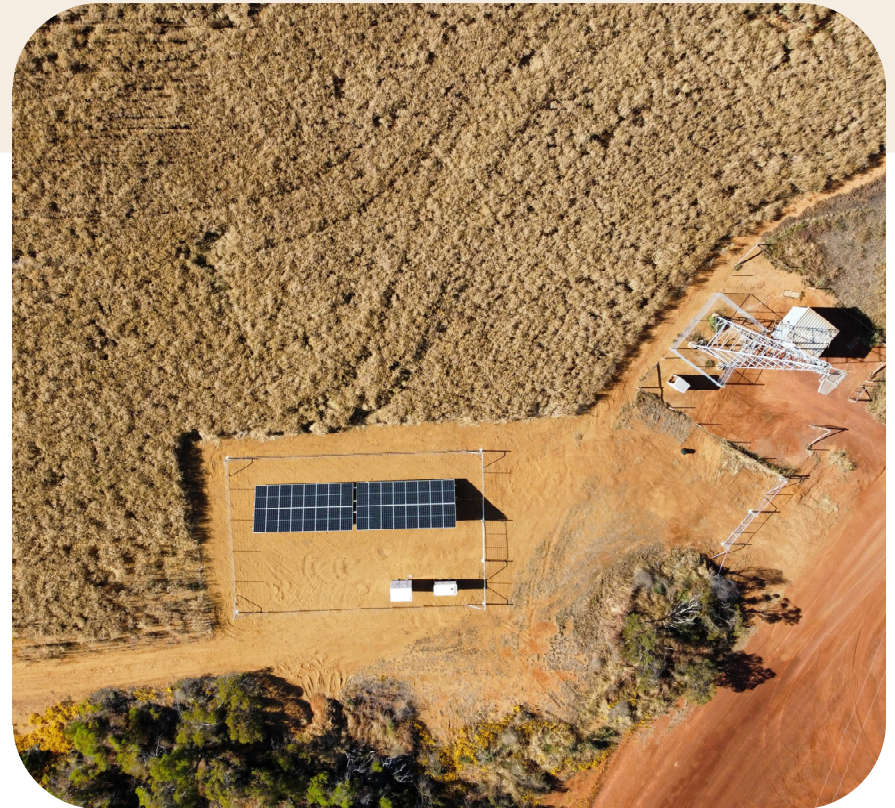
Standalone Power Systems (SAPS)
